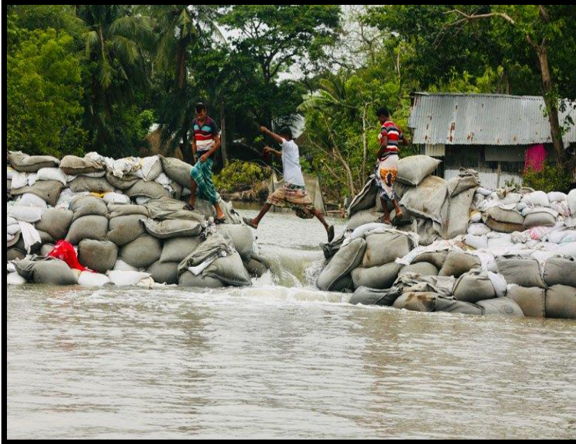
Mongla's Banishanta village embankment heavily damaged due to storm (Image source: Dhaka Tribune)
